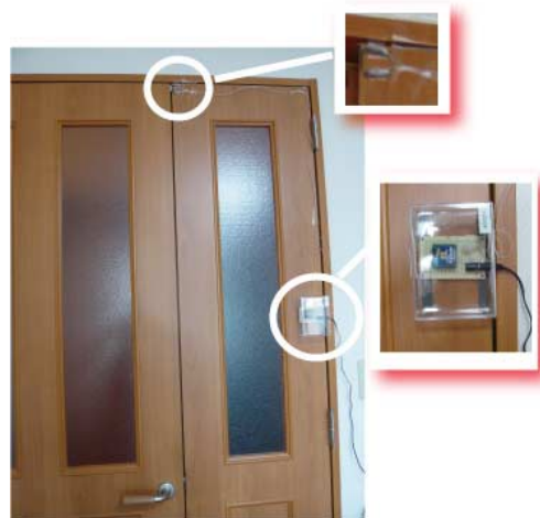
Figure 9. Sensor placement on door – House A.
